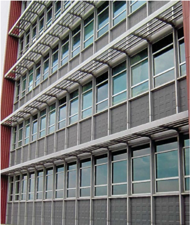
[12] This historic curtain wall features a distinctive variety of panel types which must be repaired or replicated in a restoration project if any are damaged or missing.
