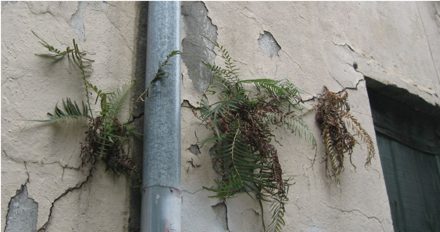
[3] Not Recommended: Cracks in the stucco have not been repaired, thereby allowing ferns to grow in the moist substrate which will cause further damage to the masonry.
