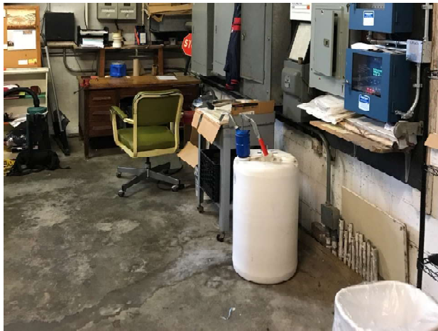
Figure 44—Concrete floor sealer worn
