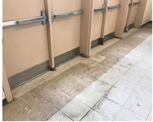
Figure 38—Stained & delaminated tile at '83 bldg.
