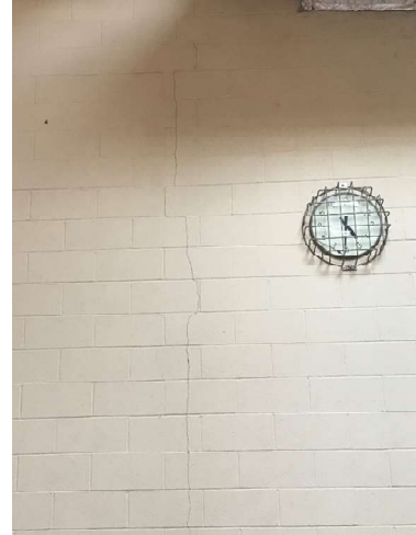
Figure 49—Crack in Gymnasium wall
