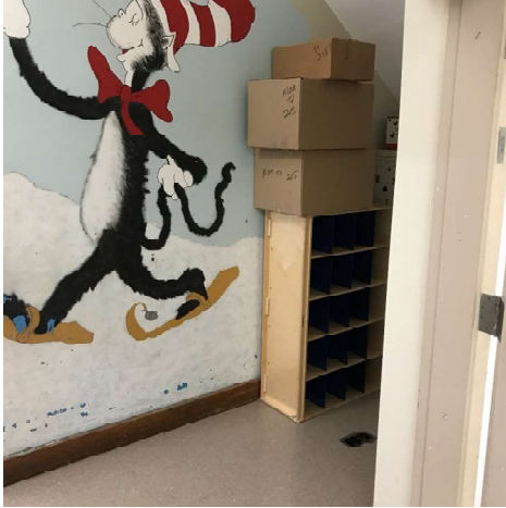
Figure 37—Delaminated & damaged VCT
