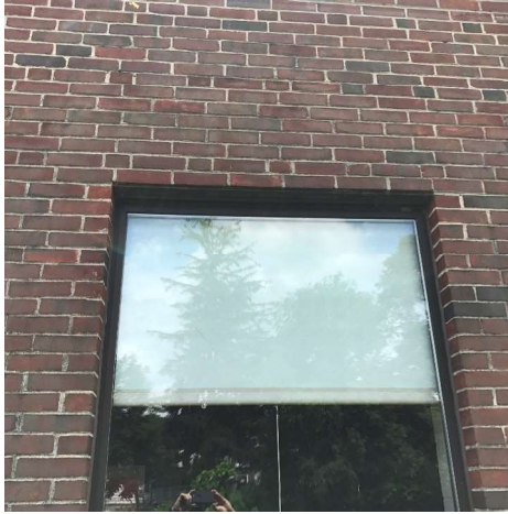
Figure 16—Non Low-E coated window glazing
