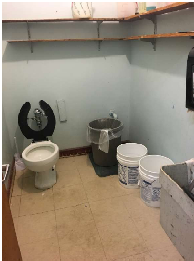
Figure 3 — Toilet and Janitor's Sink
