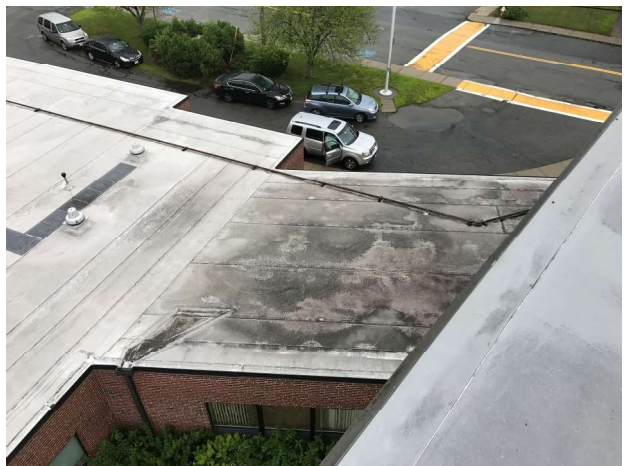
Figure 36– Poor drainage at link to '52 building
