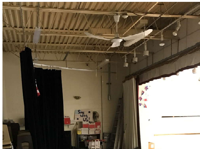
Figure 72—Stage / Platform rigging
