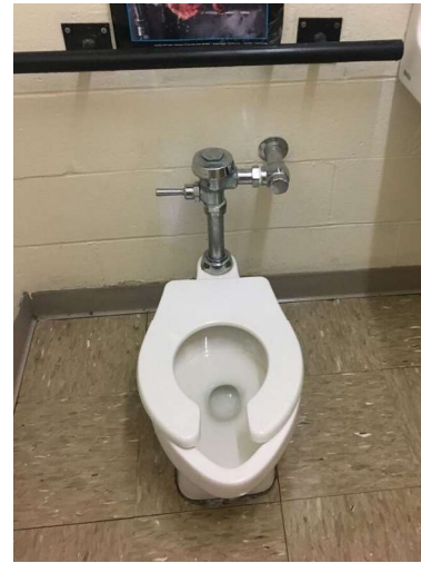
Figure 2— Small pre-k toilet
