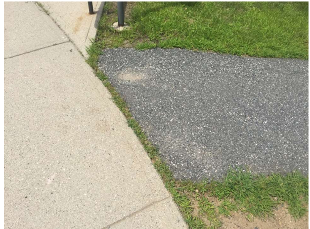
Figure 34—Gap at union of sidewalk materials
