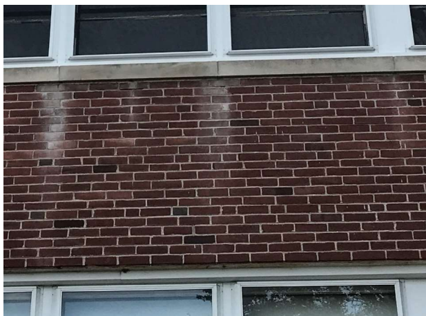
Figure 20—Failing sealant stains on brick
