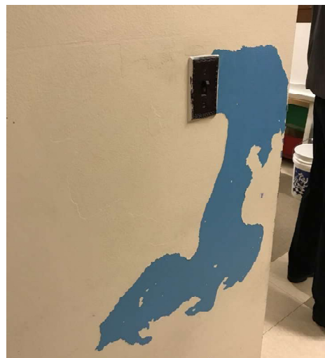
Figure 53—Paint peeling of plaster and lath wall
