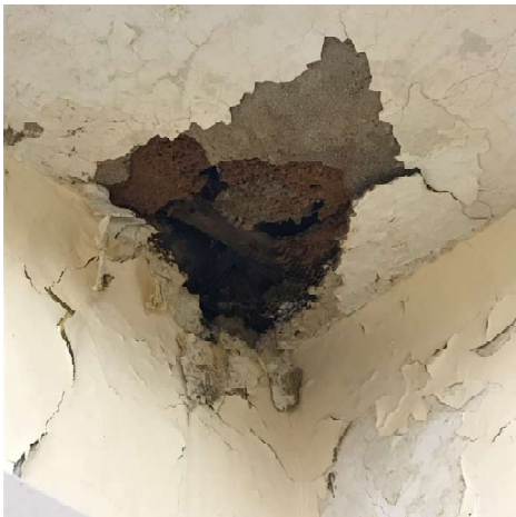
Figure 56—Water damaged ceiling 1st floor.
