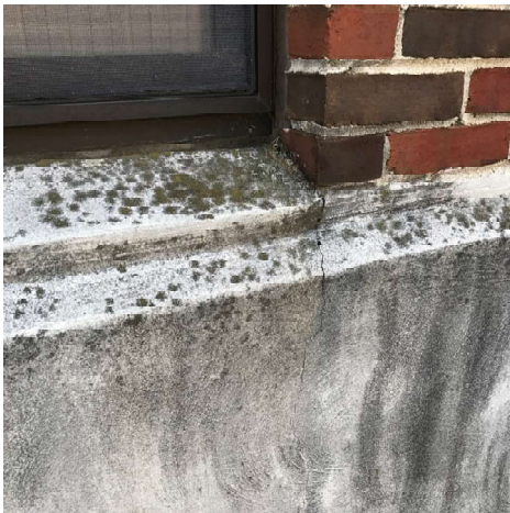
Figure 8—Crack at precast concrete window sill
