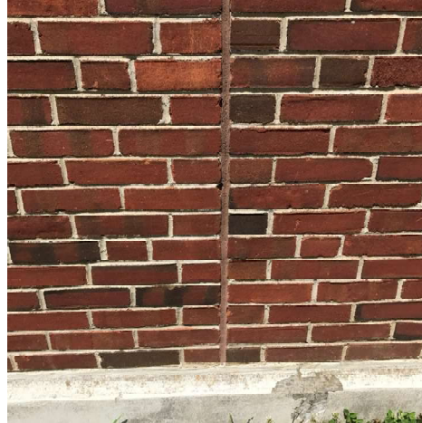
Figure 15—Dried out expansion joint caulking
