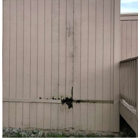
Figure 13—Rot at exterior wall of modular classrooms
