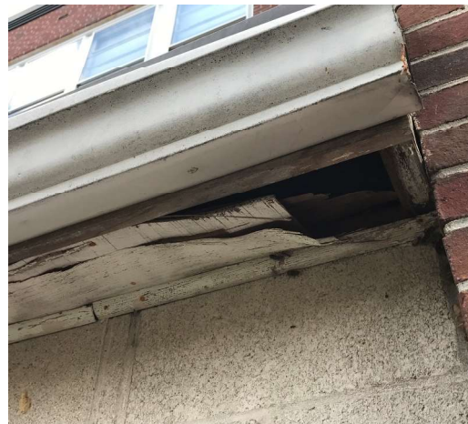
Figure 11—Rotted soffit at garage
