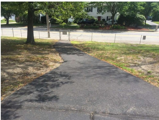
Figure 35—Steep slope at schoolyard access walkway
