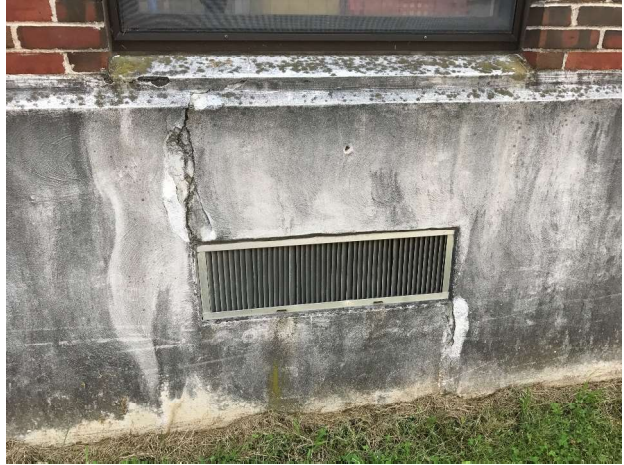
Figure 2—Cracking at unit vent grille
