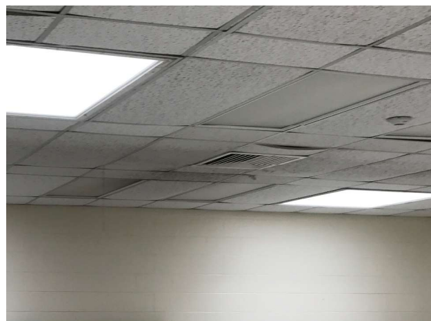
Figure 59—Soiled ceiling panels at return grilles
