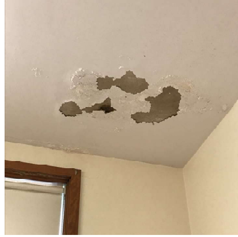
Figure 55—Flaking ceiling paint & water damage
