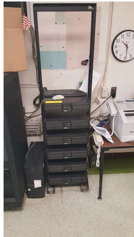
Figure 7- UPS Rack for PA System
