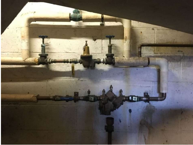
Figure 5— Backflow preventer and PRV (HVAC)
