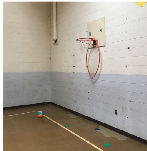
Figure 40—Worn down paint on Gymnasium floor
