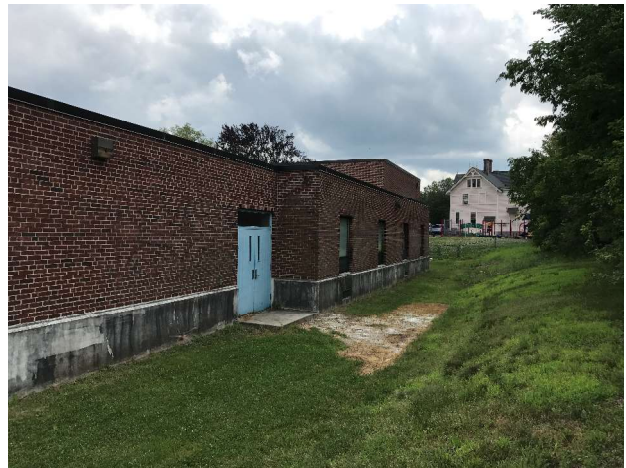
Figure 4—Typical non-accessible side door
