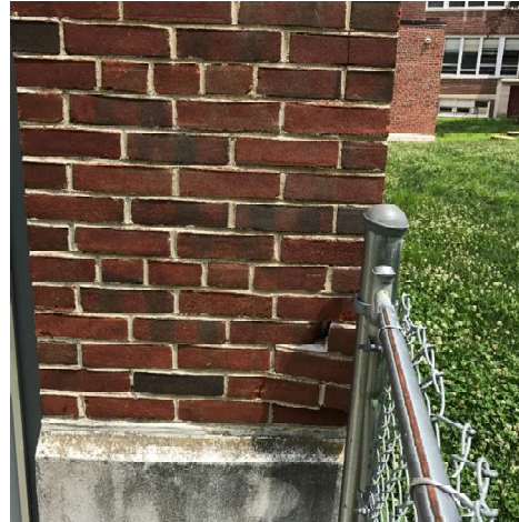
Figure 7— Cracked and displaced brick NW corner
