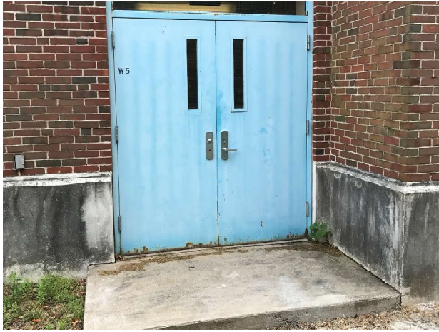
Figure 6—Exit stair discharge door with step
