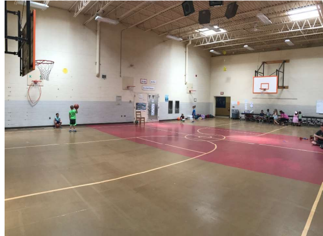
Figure 70—Lack of wall pads at gymnasium
