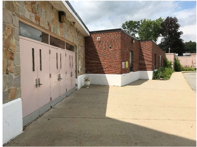
Figure 2—Non-accessible entrance no curb cut ramp
