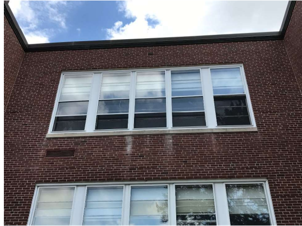
Figure 28—Degraded paint on louvers @ '52 building
