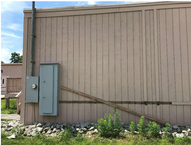
Figure 14—Trim board fallen of side of modulars
