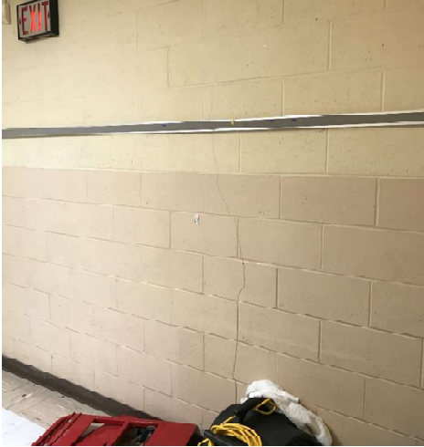
Figure 48—Crack in corridor of '83 addition
