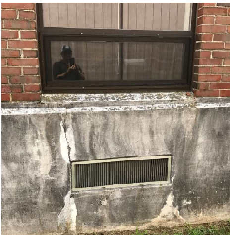
Figure 3—Cracking at unit vent grille
