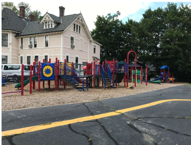
Figure 5—Playground surface and equipment issues
