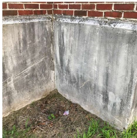
Figure 5—Discolored and dirty foundation wall
