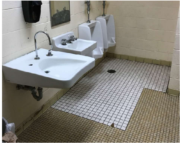
Figure 43—Large area of mismatched tile
