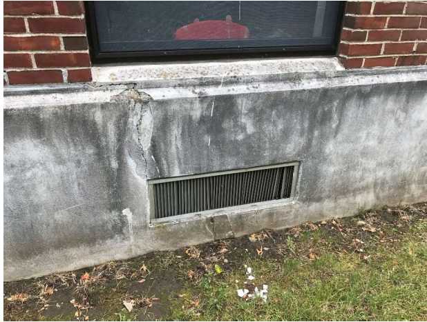
Figure 27—Damage at '83 addition.
