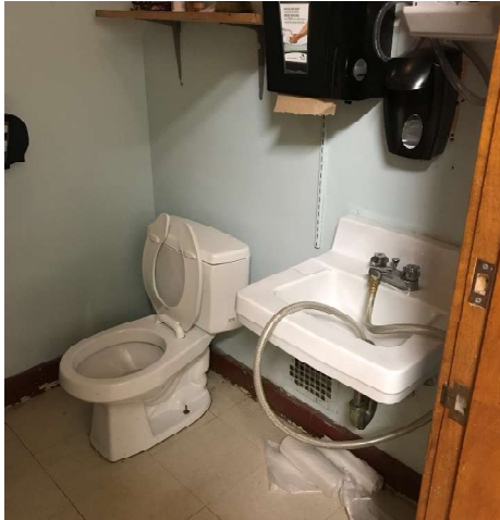
Figure 10—Non accessible toilet room.
