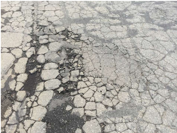
Figure 27—Poor condition of bituminous concrete
