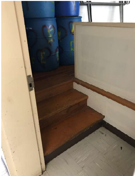
Figure 8—Stair at side of stage / platform
