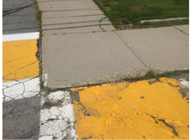
Figure 32—Excessive gap at crosswalk and sidewalk
