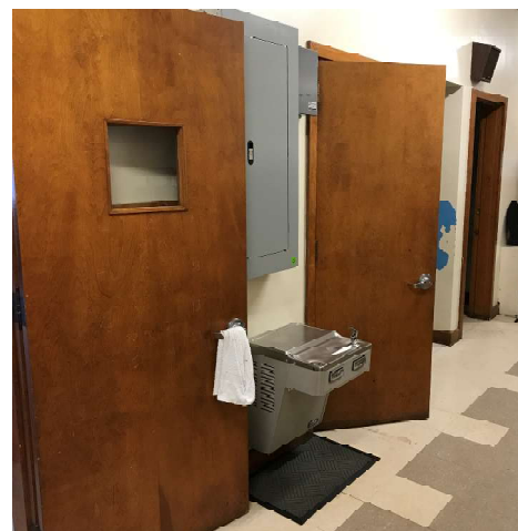
Figure 15—Non-accessible drinking fountains
