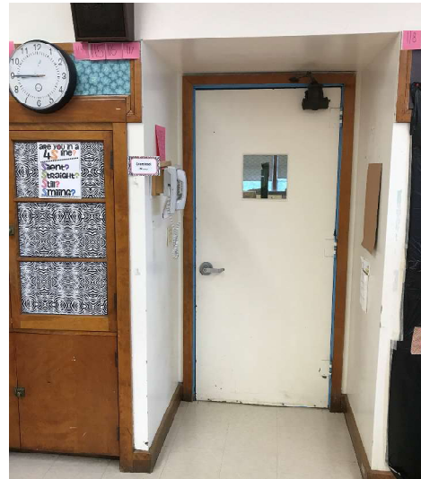
Figure 19—C.R. door lacking pull side clearance
