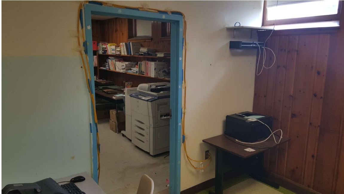
Figure 1-IDF showing insufficient power distribution for equipment
