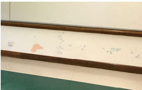
Figure 52—Paint peeling at plaster and lath wall
