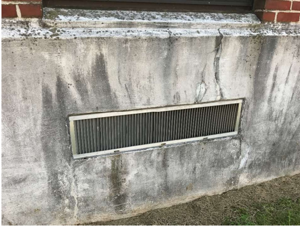
Figure 1—Cracking at unit vent grille
