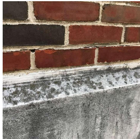
Figure 9— Degrading mortar joints typical
