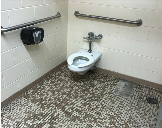
Figure 42— Area of missing mosaic tile
