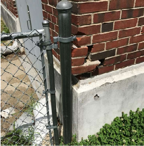
Figure 6—Cracked and displaced brick NW corner
