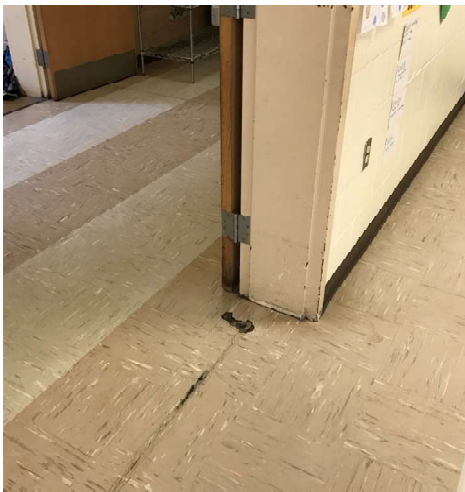
Figure 39—Worn down VCT tile at door '83 bldg.
