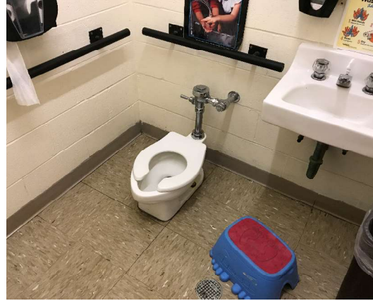
Figure 17—Non-accessible classroom toilet
