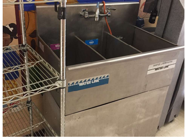
Figure 2—Three bay sink
