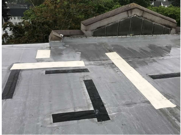
Figure 32– Patches on '52 building roof
