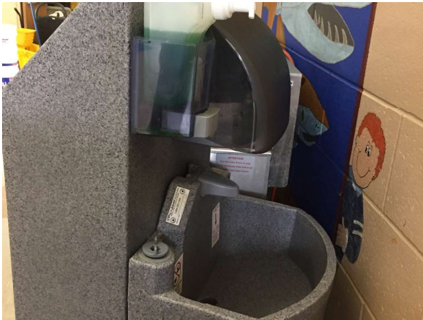
Figure 3—The hand washing station
