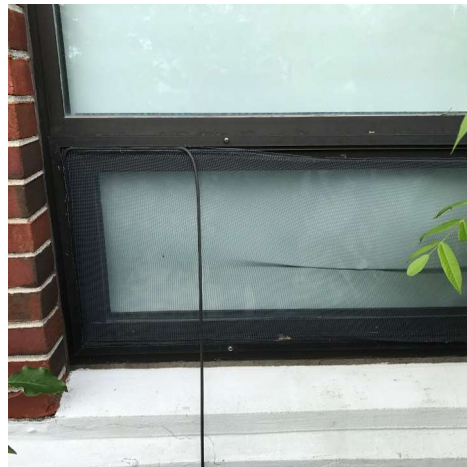
Figure 19—Loose screening and splines
