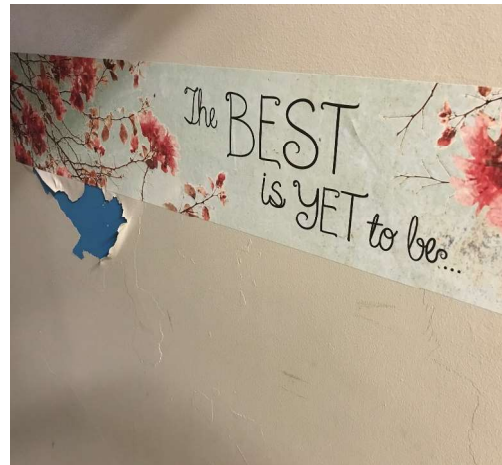
Figure 51—Paint peeling of plaster and lath wall
