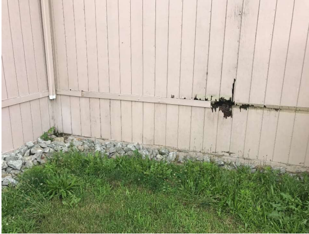
Figure 12—Rot at exterior wall of modular classrooms
