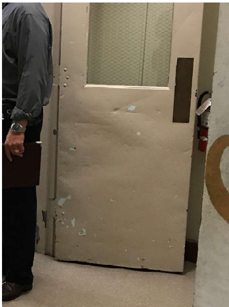
Figure 62—Damaged face of HM door
