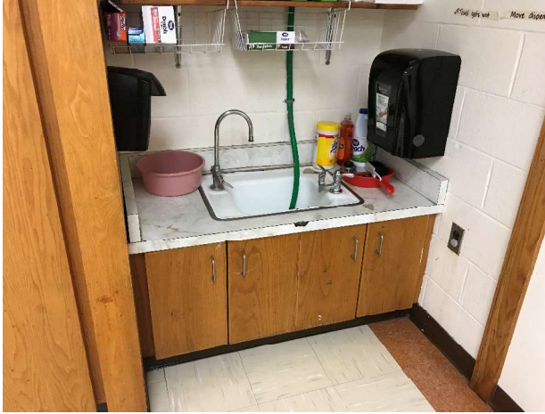
Figure 16—Typical non-accessible sink in classroom
