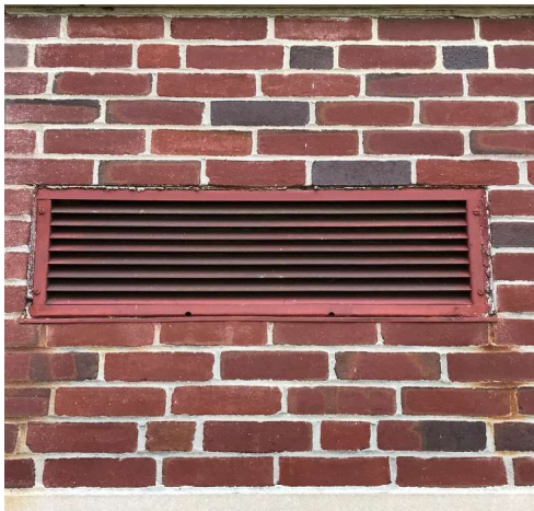
Figure 29—Degraded caulking around lower typical
