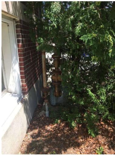
Figure 7— Gas service and meter
