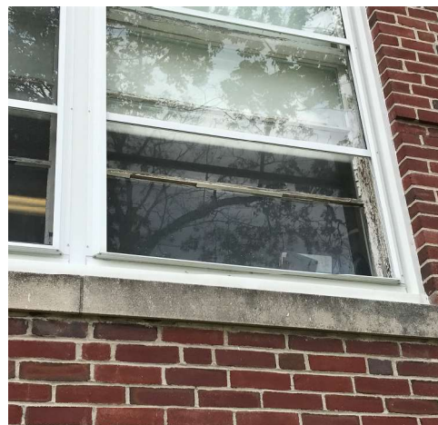
Figure 21—Deteriorating wood windows '52 bldg.
