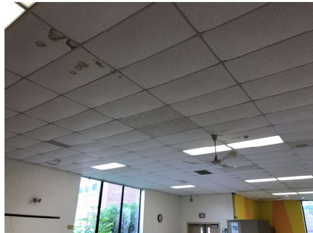
Figure 57—Sagging & stained ceiling panels.
