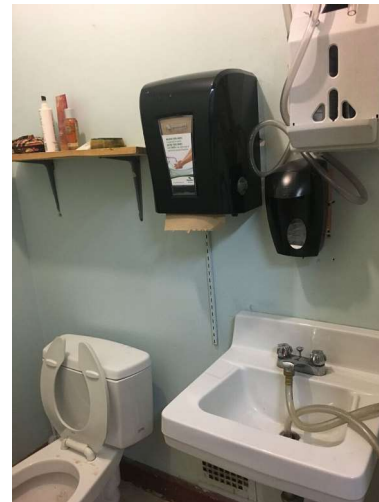
Figure 4—Tank type toilet and chemical dispenser
