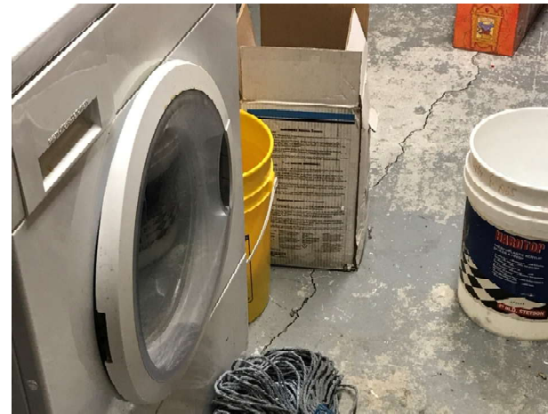
Figure 45—Sealed concrete floor worn away typical
