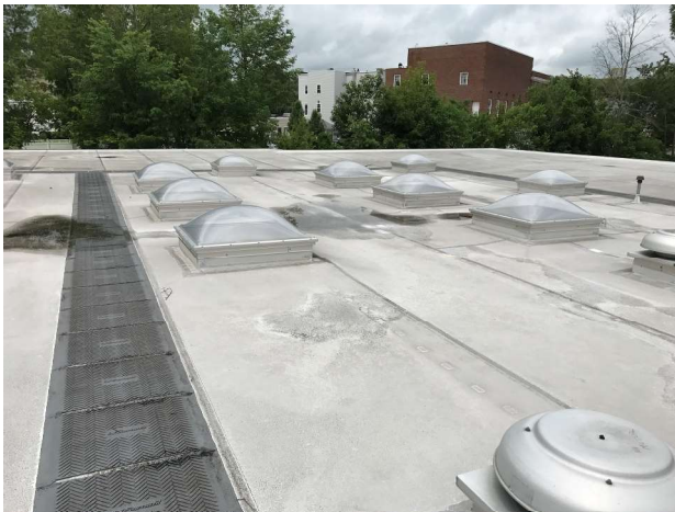
Figure 33– Areas of minor ponding on '83 roof
