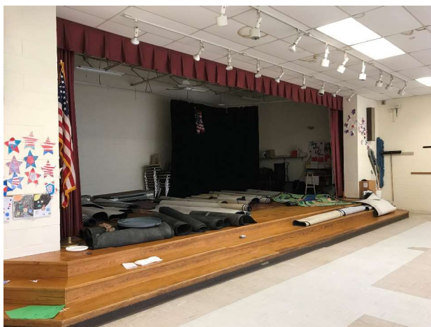
Figure 46—scuffed and gouged stage floor
