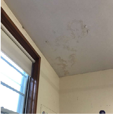
Figure 54—Flaking ceiling paint & water damage
