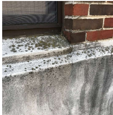
Figure 4—Discolored and dirty foundation wall
