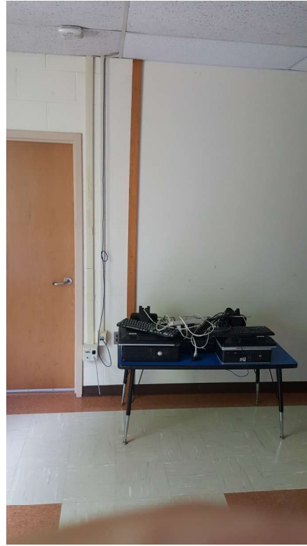
Figure 15– Computers in Classrooms Wireless AP Above
