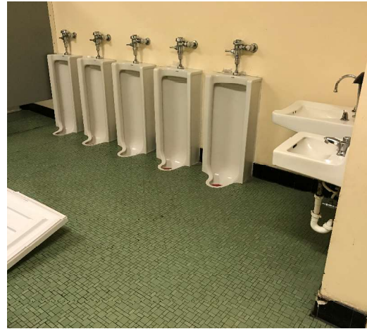
Figure 11—Non accessible gang bathroom typical
