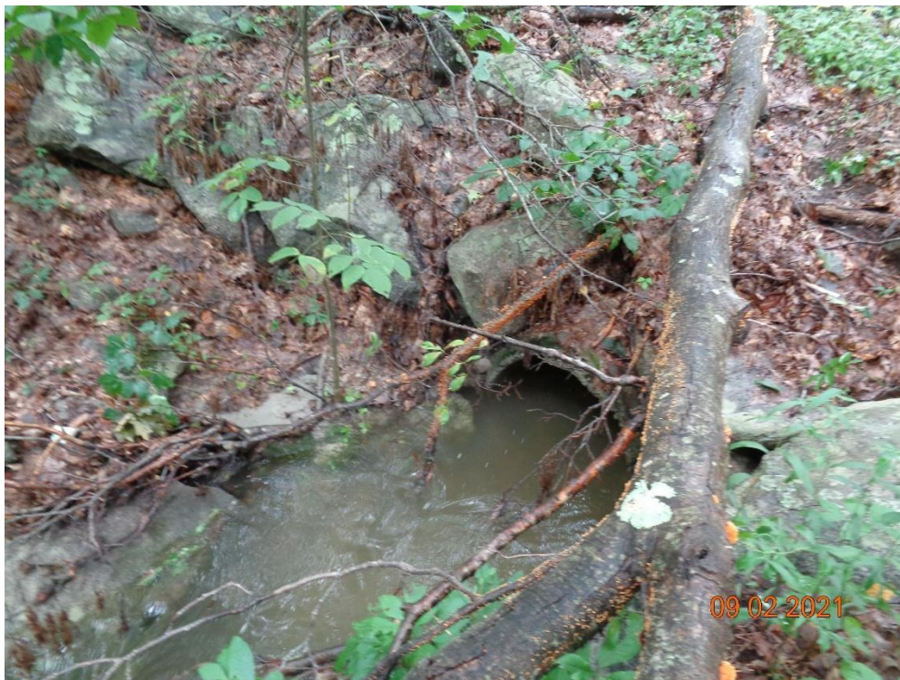
Photo 6: Outlet of the Leland Road drainage system near the intersection of East Street.
