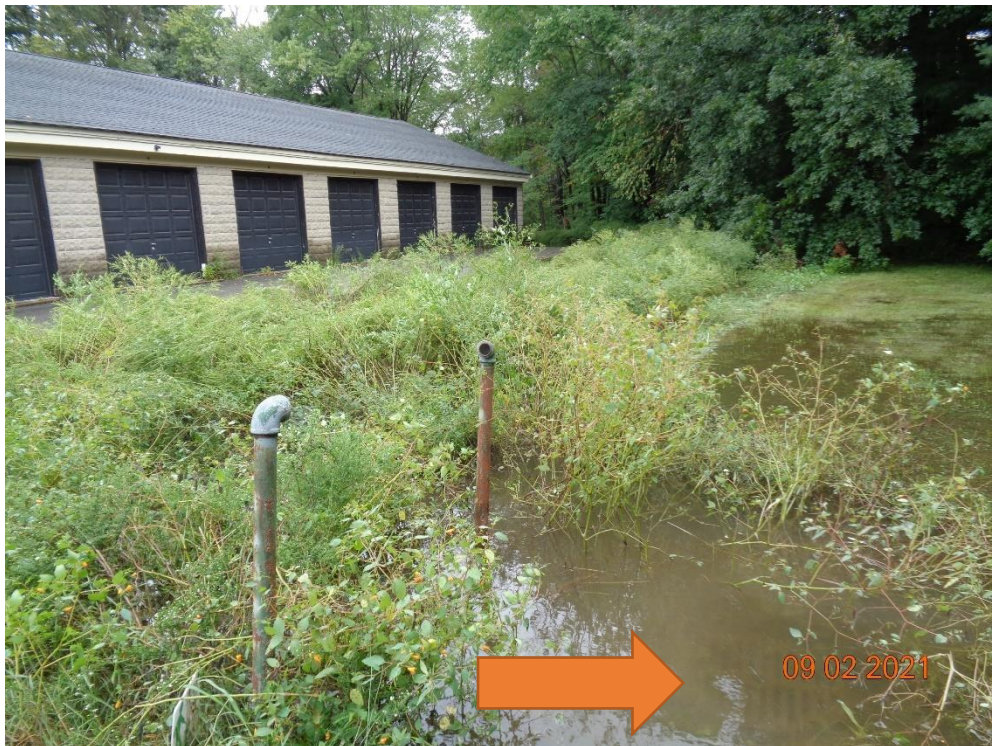
Photo 4: Submerged catch basin grate behind #11 Leland Road.
