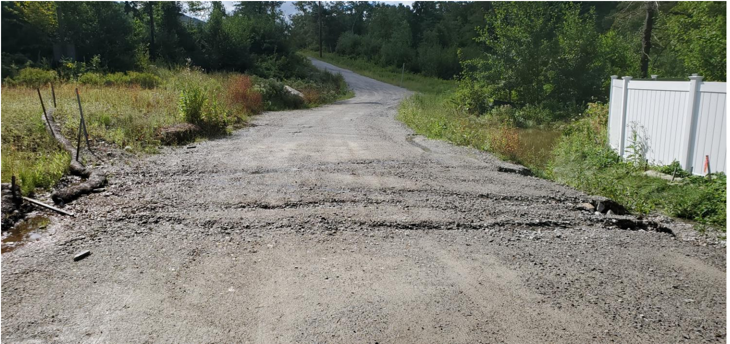
Scouring across the Syncarpha I access road from Area 6 and slumping of the edge into the drainage swale.
