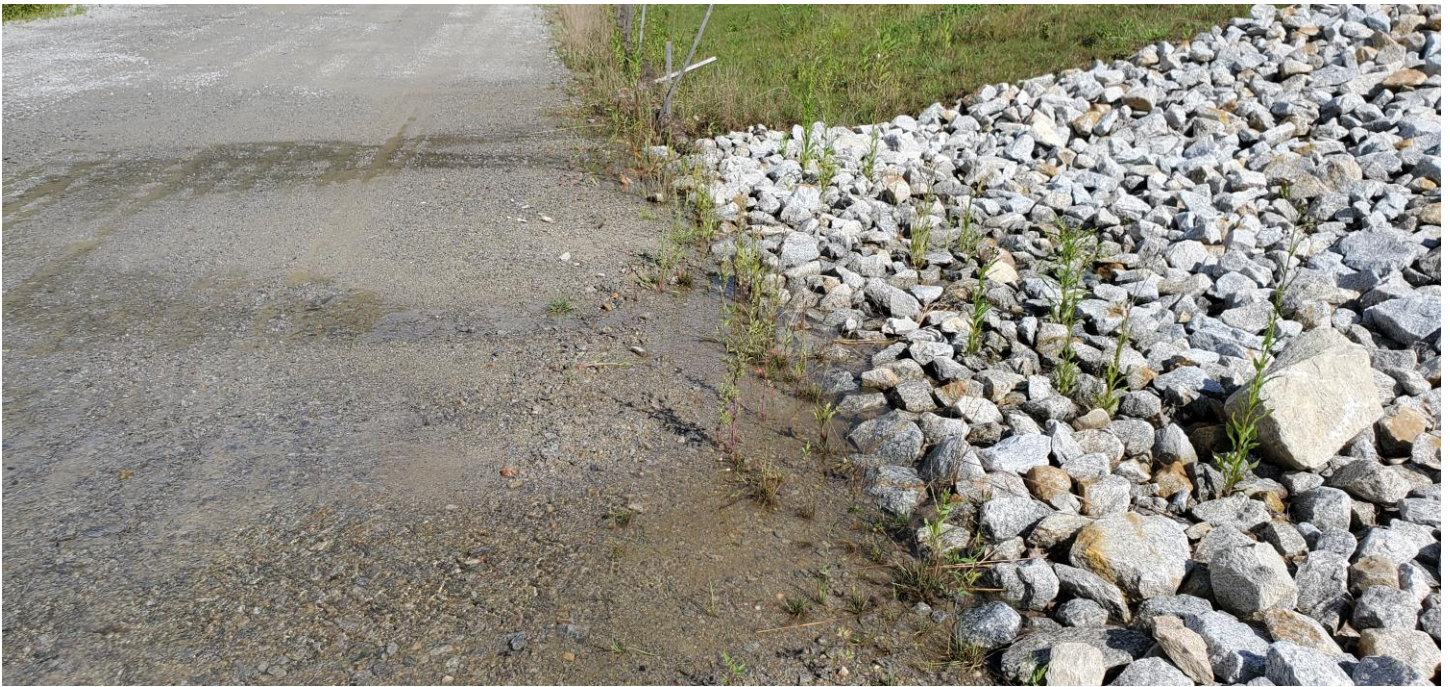
Water discharging from the base of the emergency spillway from the Stone Hill infiltration basin and flowing across the Syncarpha 1 access drive.
