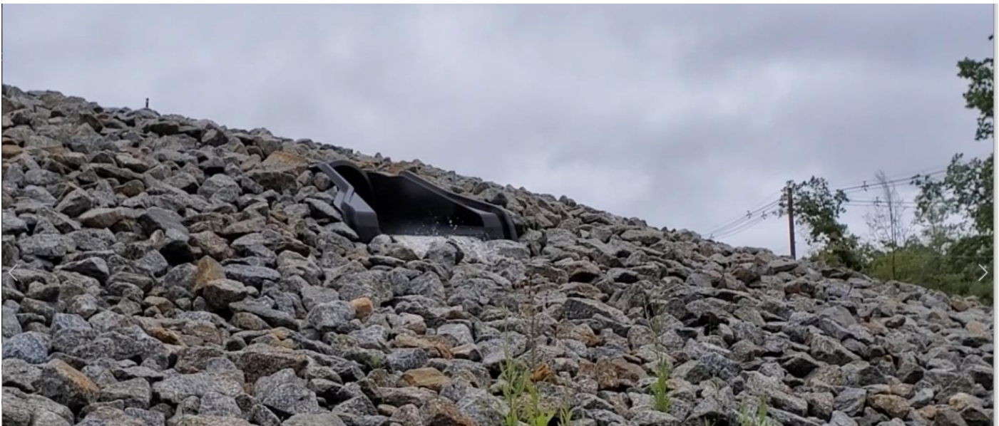
Water flowing out of the outlet from the Upper Infiltration Basin at Stone Hill.
