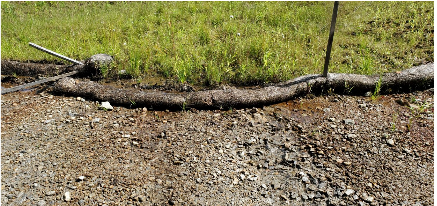
Breakout/shallow flow emanating from graded areas on Stone Hill site.
