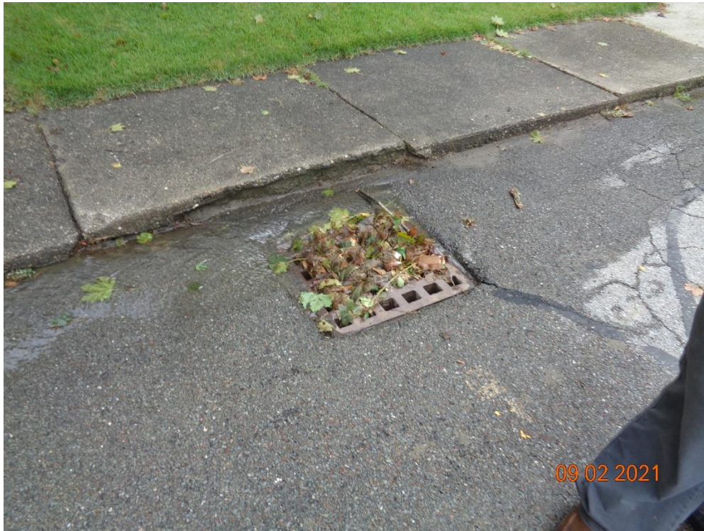
Photo 3: Catch basin near #21 Leland Road that received overland flow from the backyards.
