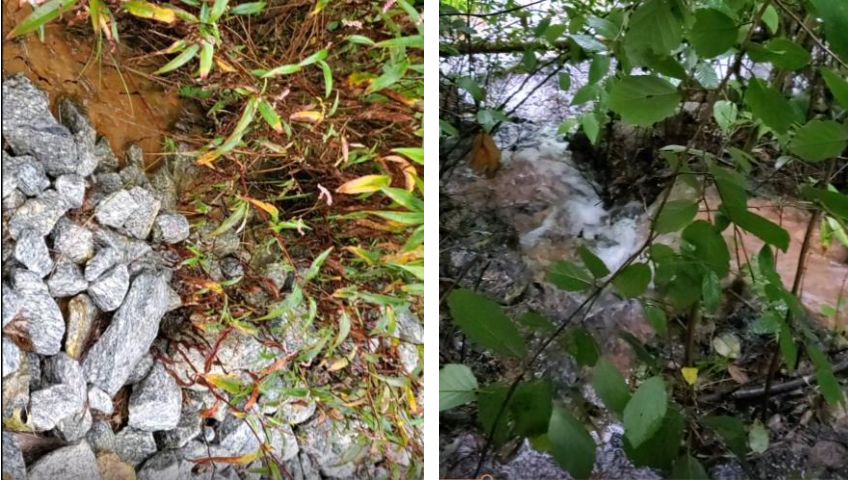
Photos of concentrated flow emanating from the base of the riprap slope on the north side of upper infiltration basin.
