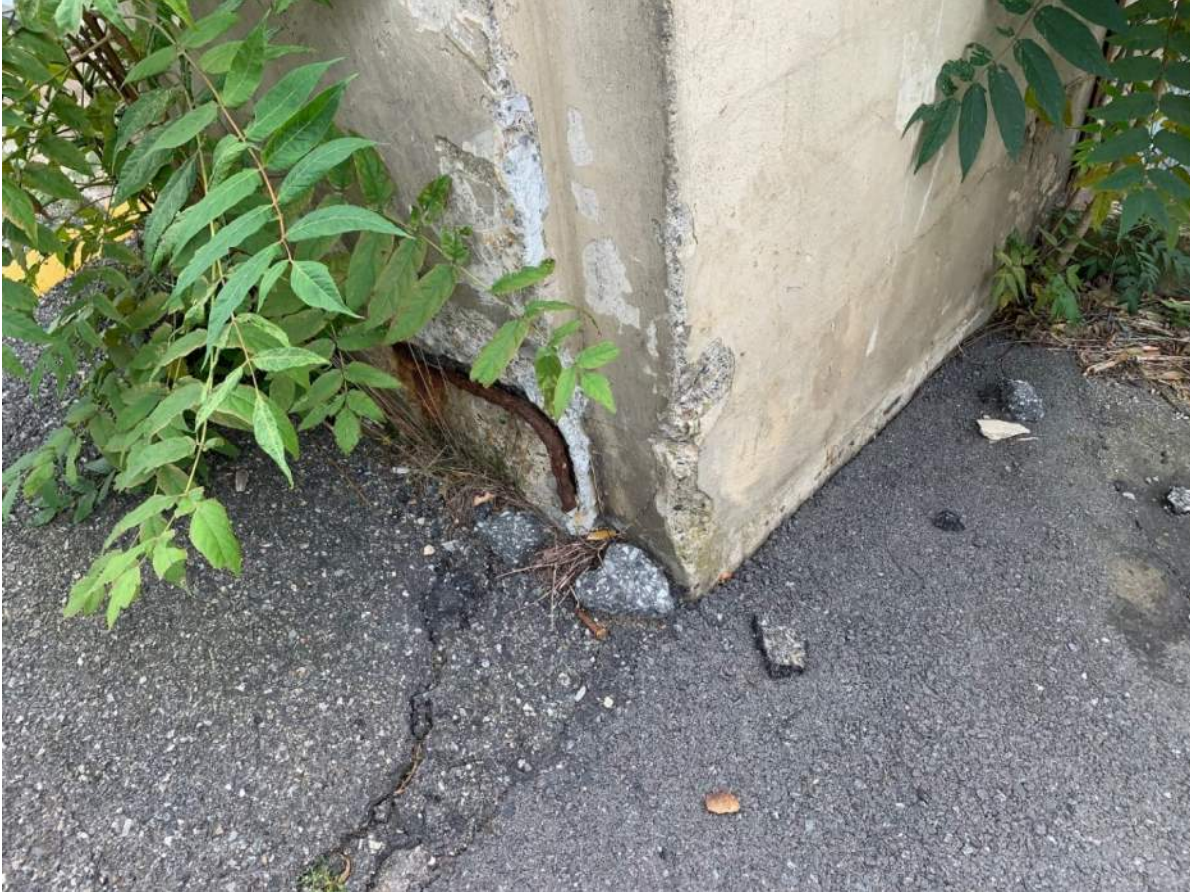
Photo #14: Close-up view of exposed rebar at base of foundation wall near northwest corner of building.
