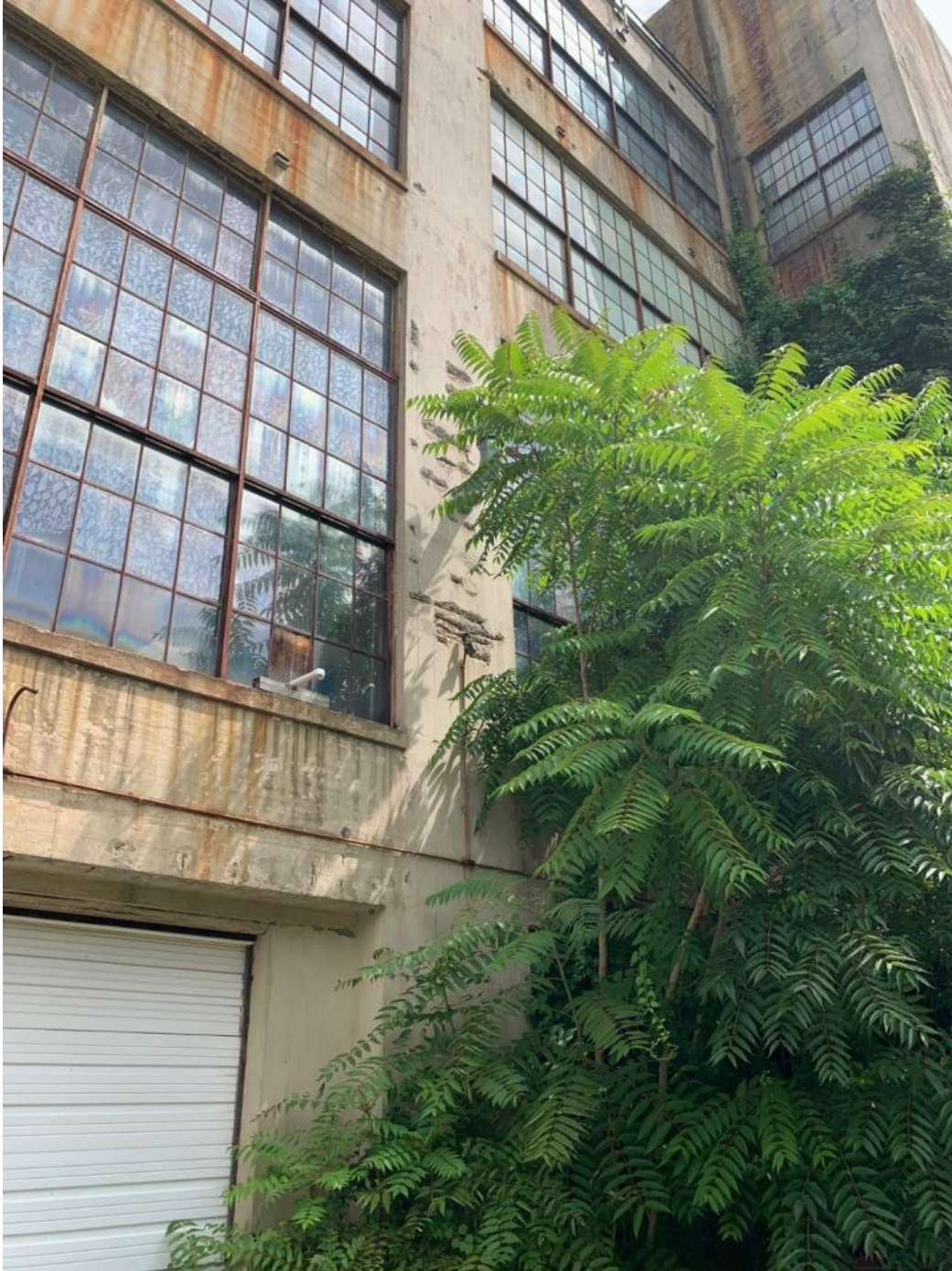
Photo #10: View of rear wall of building showing spalls in concrete and exposed rebar.
