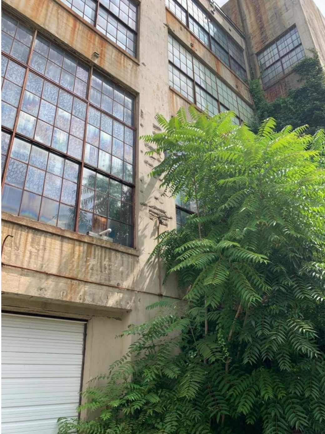
Photo #10: View of rear wall of building showing spalls in concrete and exposed rebar.
