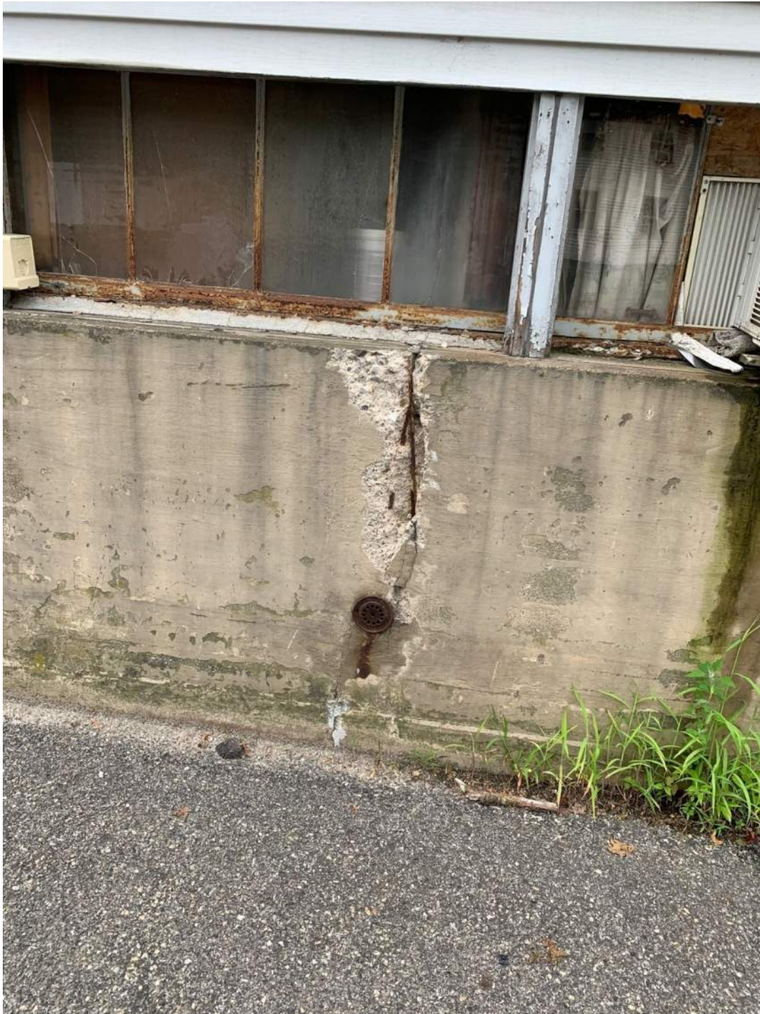
Photo #13: Close-up view of significant crack and spalled concrete in foundation wall. Structural repairs to these types of cracks and spalls will be required.
