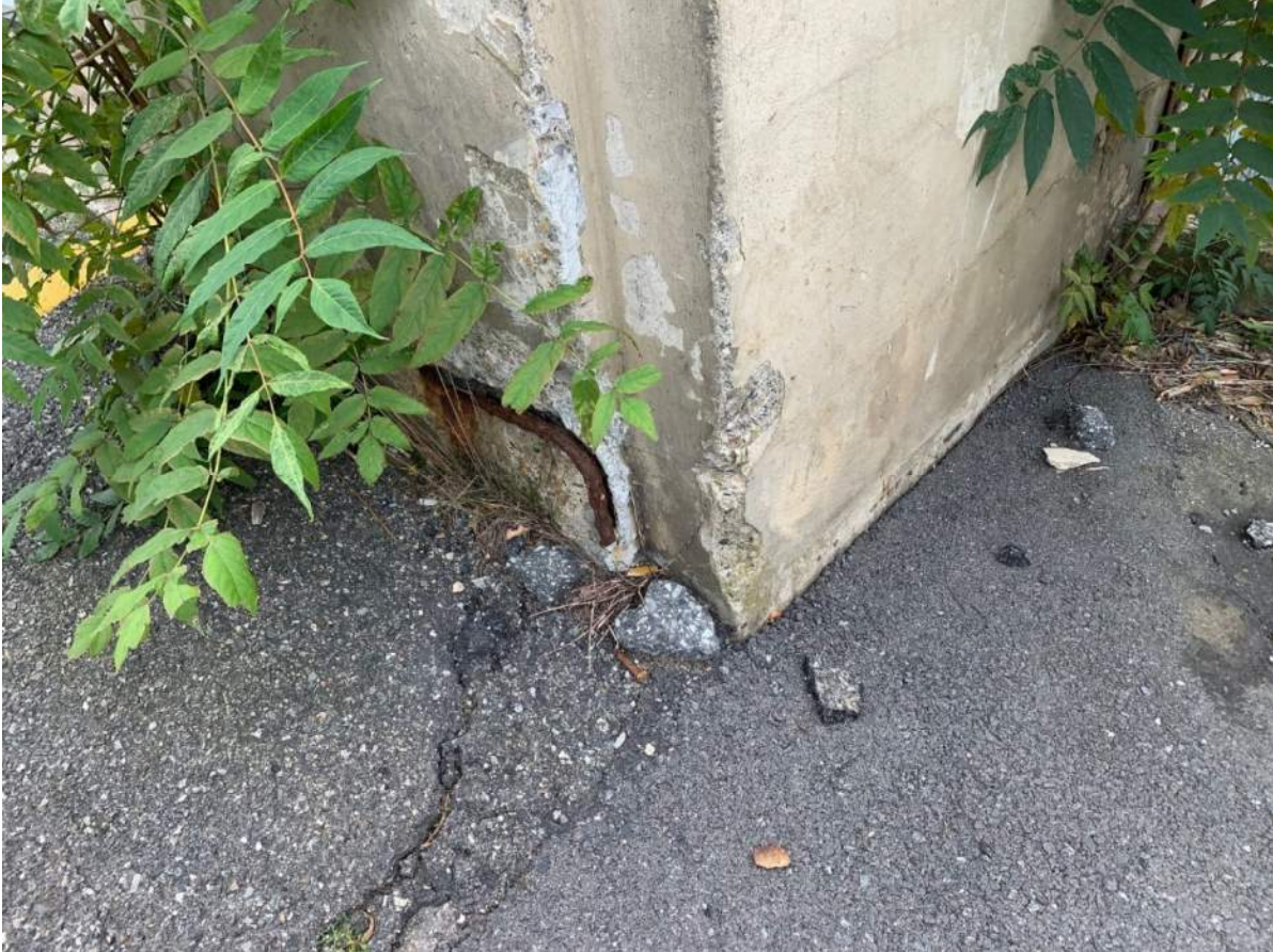
Photo #14: Close-up view of exposed rebar at base of foundation wall near northwest corner of building.
