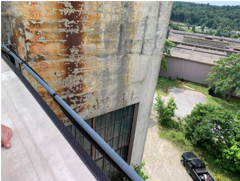
Photo #7: View of concrete wall on west side of freight elevator enclosure where rebar in wall is exposed and has spalled the surface of the concrete.
