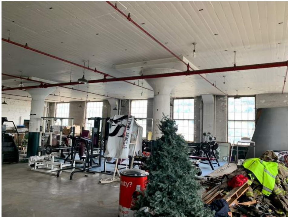
Photo #4: View of reinforced concrete column, column capital, drop panel and two-way structural slab at underside of upper floor level.
