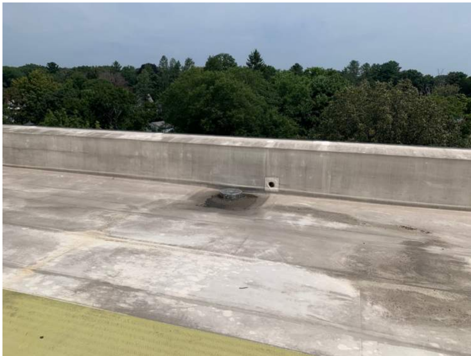
Photo #5: View of roof and short parapet along north side of building.
