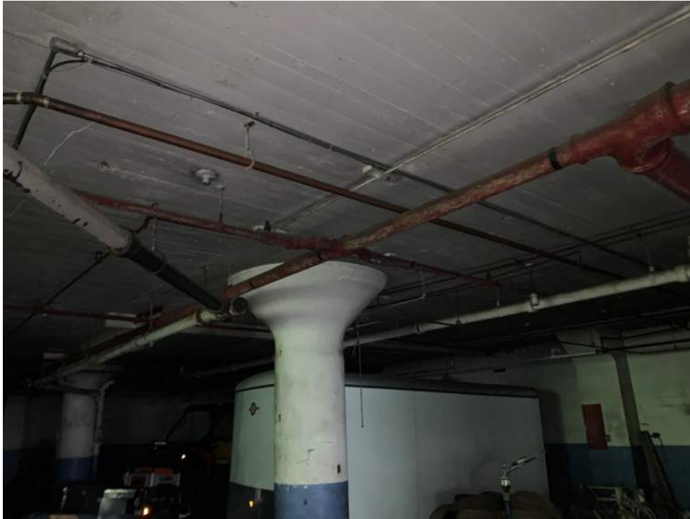
Photo #2: View of underside of Level 1 slab standing in basement showing interior reinforced concrete column, column capital, and underside of two-way concrete slab. The underside of the Level 1 slab does not have any drop panels.
