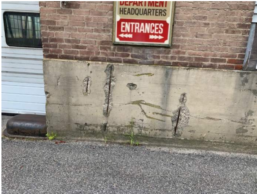
Photo #11: View of foundation wall along Main Street showing exposed rebar and spalled concrete.
